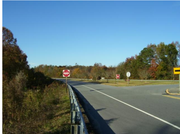
Guard rails installed by NC Department of Transportation along U.S. Highway 13 at the NW 2 nd Street intersection
